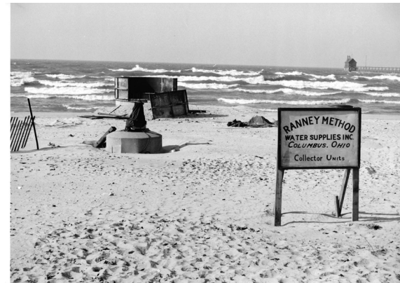
Pictured above is the City of Grand Haven's installation process of the retired 1950's Ranney Well Collectors (one of three). Designed to deliver 7 million gallons per day (MGD), but only could deliver 5 MGD. All three wells were removed in 2002.
